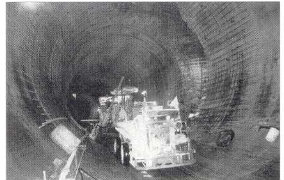
TUNNEL VISION: The plaintiff was injured in a January 1996 accident at this deep tunnel project located in Morton Grove, Ill.
